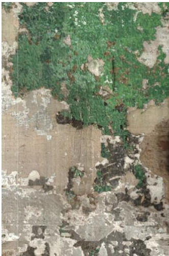
At Eastham Prison, a handheld scanner captured images of peeling paint.
